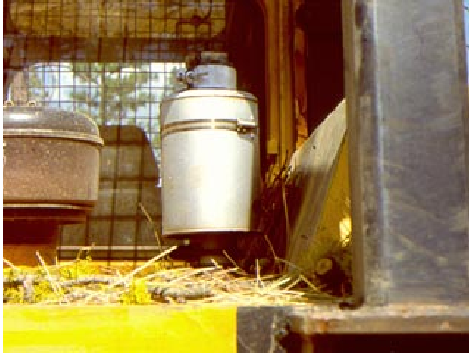
Photograph 4-12. Accumulated Flammables Around Exhaust
