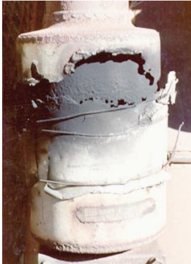
Photograph 9-8. Leaking Exhaust System
