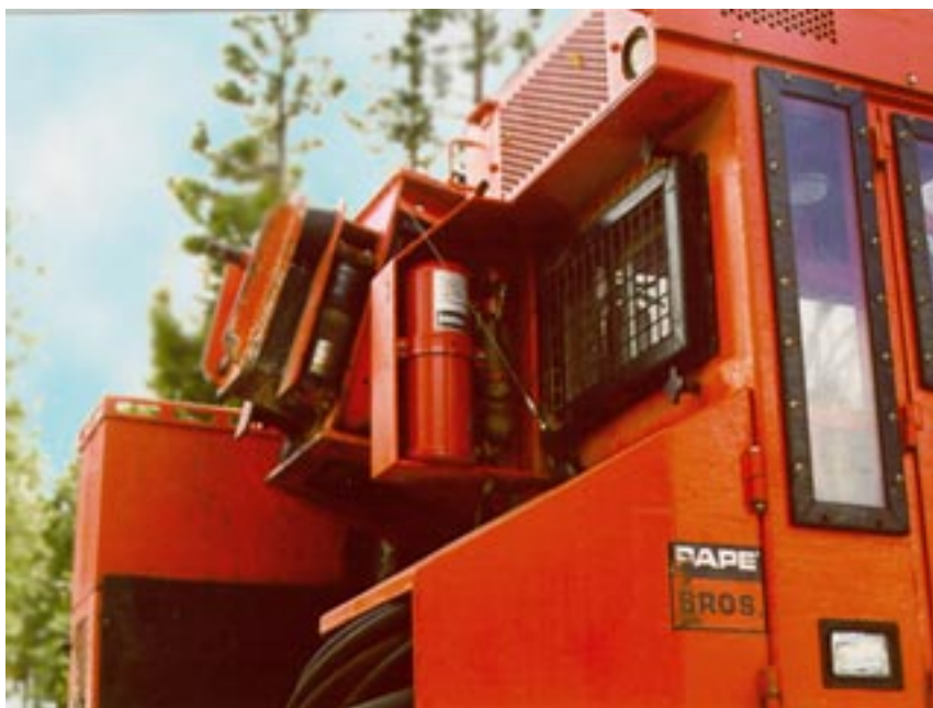
Photograph 9-10. Fire Suppression System
