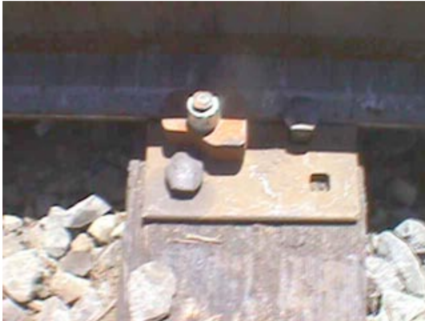
Photograph 7-1. Rail Corner Hold Down
