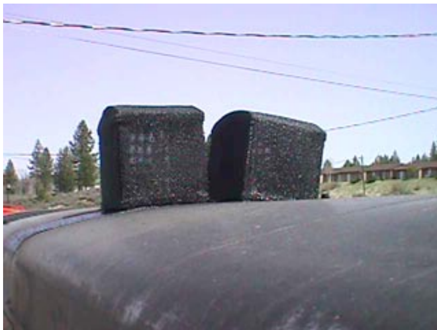
Photograph 5-3. Exhaust Stack with Illegal Screen (Requires an Approved Spark Arrester)
